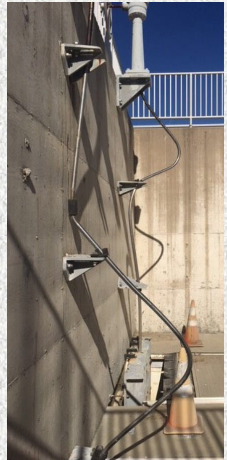
Excessive force applied to bound gates caused stems to bend.
