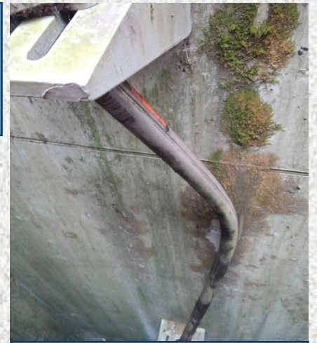
Failed limit switches and missing stop nut caused stem to bend.
