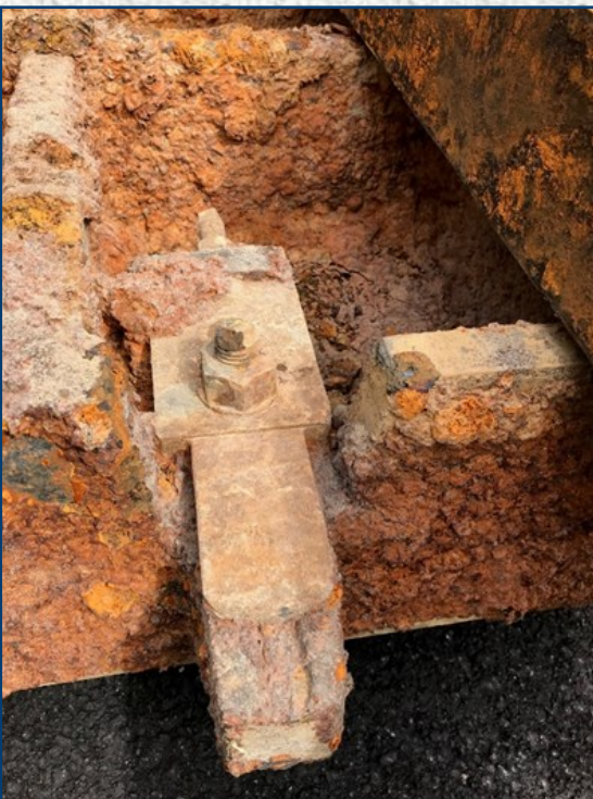
Condition of bottom wedge upon arrival at Quabbin.
