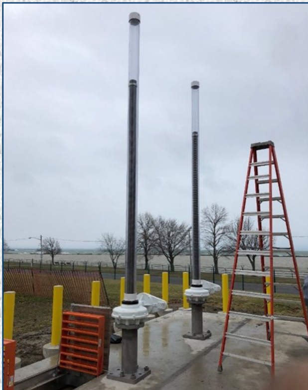
Pedestals, gear boxes, stop nuts, operator stems and stem covers after installation.
